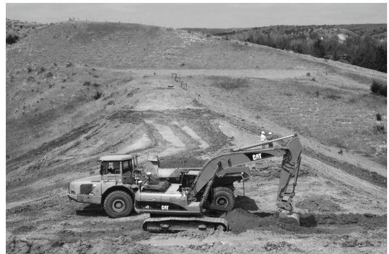
The scraper shown above removes soil from the top of the structure and moves it to a storage location for later use.
