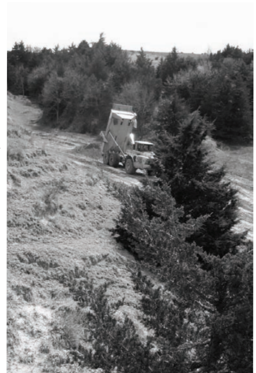
A dump truck dumps soil taken from the flood control structure to a storage area.
